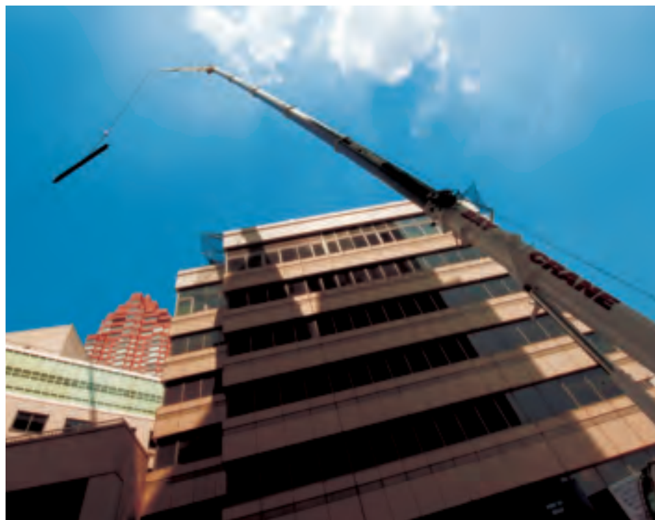
Expansion of the Hospital's East Wing began with the raising of steel this summer.
